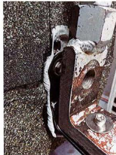
Figure 4c. Bolt failure mode.
