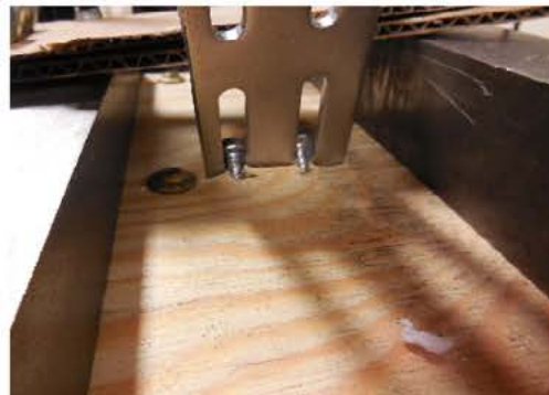
Photo 4: Closeup of Fastener Pullout
