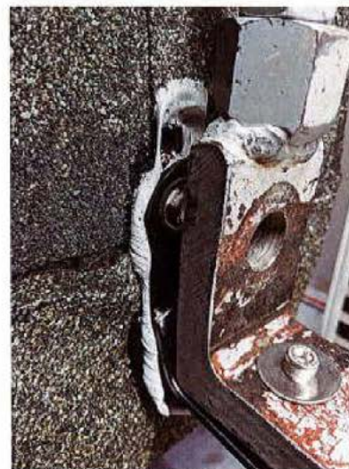
Figure 4c. Bolt failure mode.
