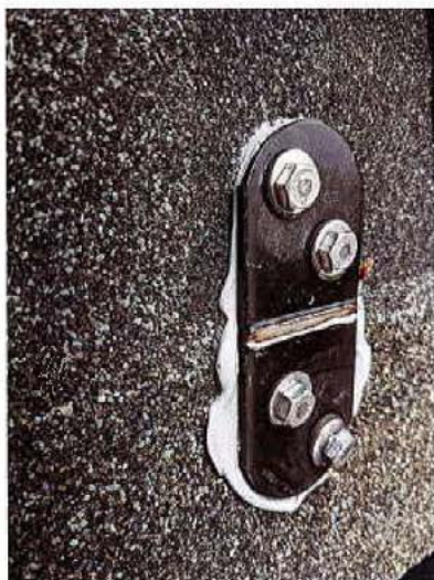
Figure 4b. Mount failure mode.
