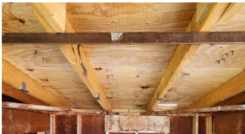
Photo No. 12 Post Test Underside
